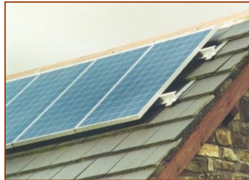
Roof mounted photovoltaic cells
