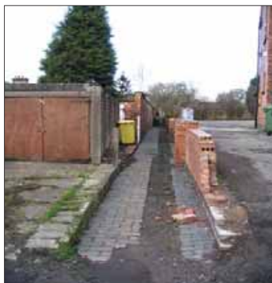
Wall to the pub car park and garages at end of terrace.
